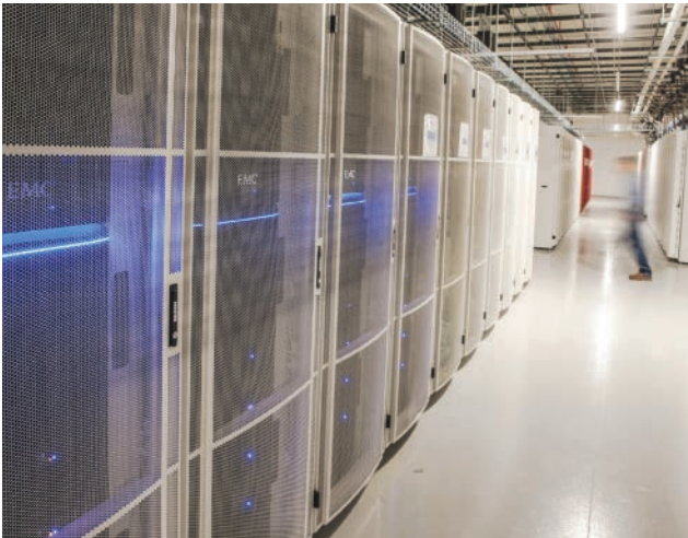
Typical Cabinet Placement. No raised floor and open plenum above.
