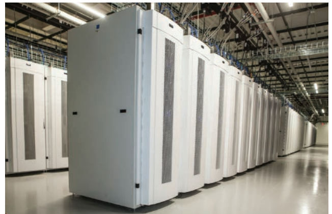
Refrigerant-based laminar cooling system located on the back panel of each rack.
